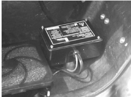
Internal electrical junction box
